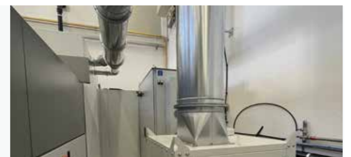
Centralised ventilation system: electronically controlled high pressure fan to effectively cool the piece.
