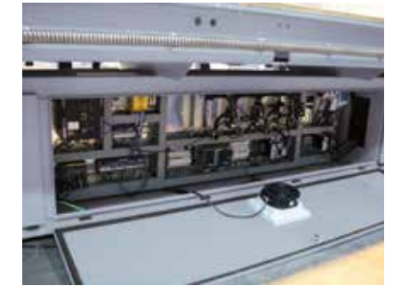
Electrical cabinet integrated into the basement
